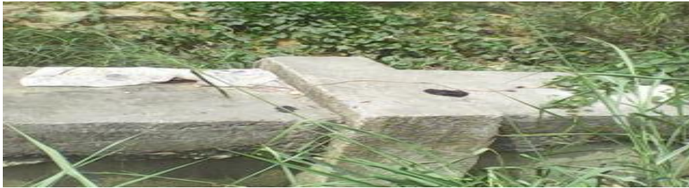
Plate 2. First section of the lined canal which convey water to the scheme
